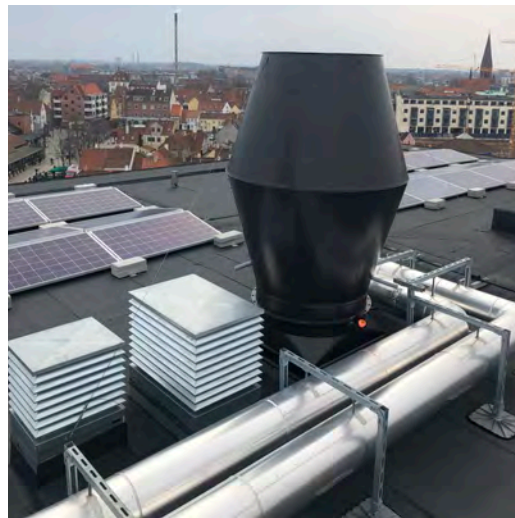
Air outlet from the kitchen
