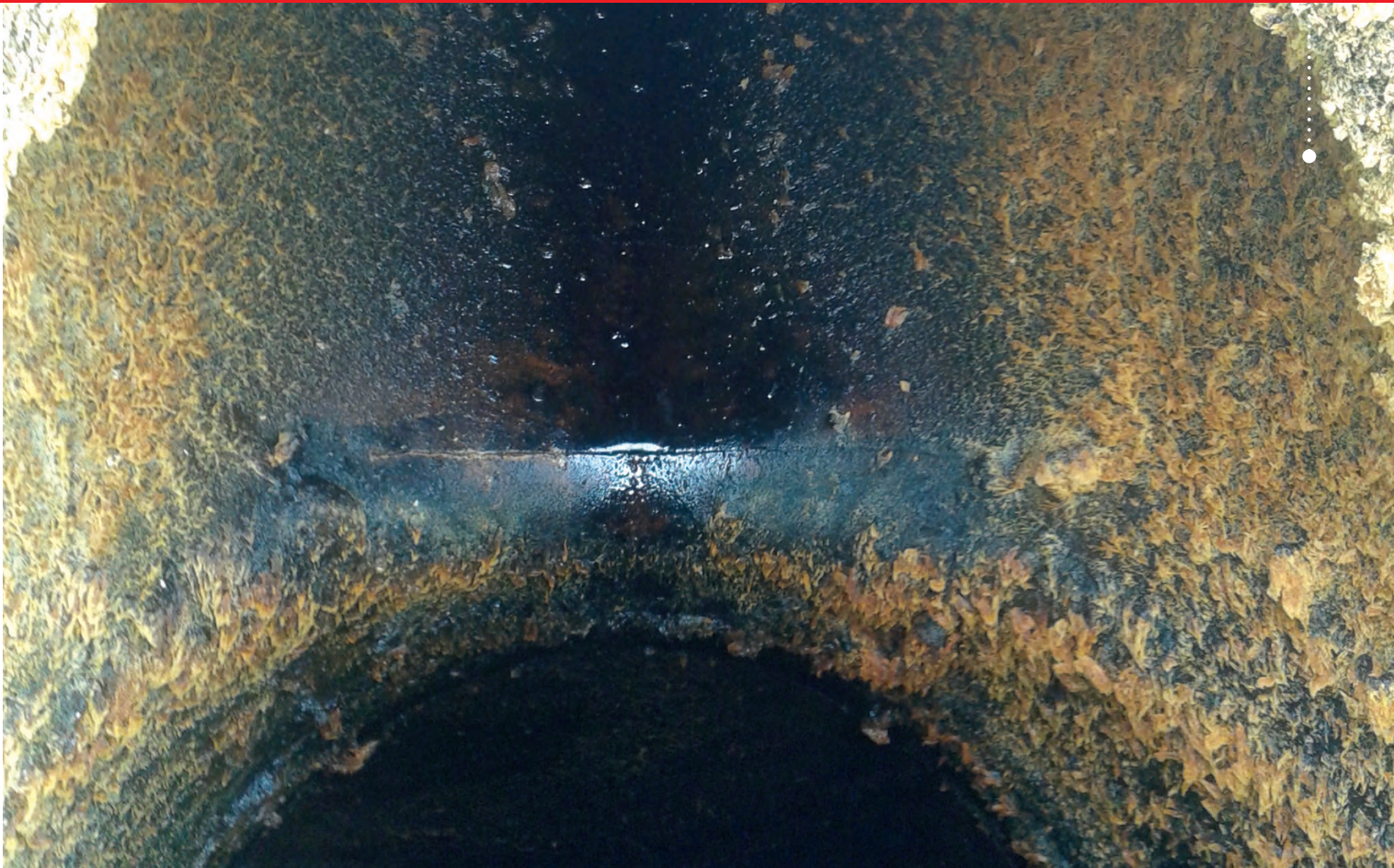
Duct without JIMCO Technology - Not cleaned for 12 months
